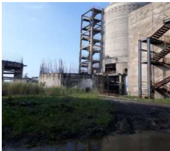
Fly Ash Silos
