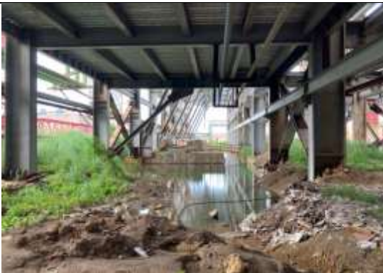
Mill area of Unit#6
