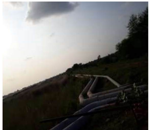
Ash disposal system
